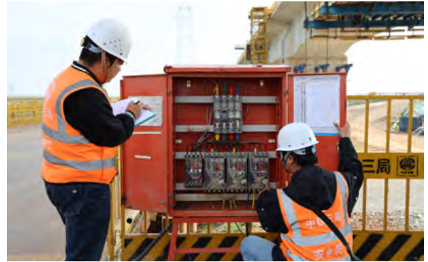
中铁三局开展消防风险隐患排查活动 China Railway No. 3 Engineering Group conducts a fire risk and hidden danger investigation
