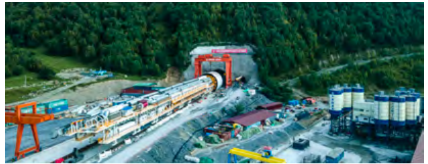
2024年4月23日，格鲁吉亚南北走廊KK公路古多里隧道贯通。 On April 23, 2024, the Gudauri Tunnel of Georgia North-South Corridor KK Highway is successfully completed.
